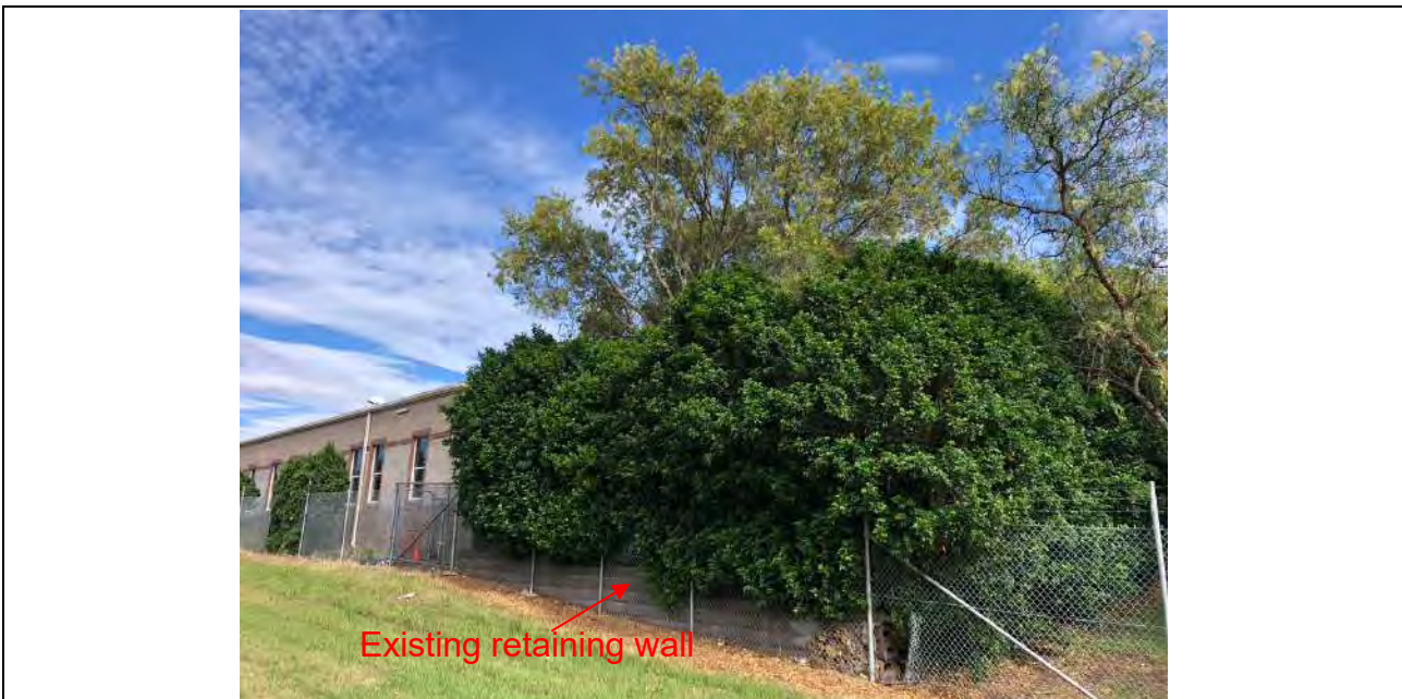
Image 2: Looking towards tree 3316, 3317, 3318, 3319 and 3320, showing the existing boundary retaining wall. The existing boundary retaining wall appears to be restricting root growth into the corridor, therefore, the proposed works within the corridor will not impact the trees. Minor canopy pruning may be required for tree 3316, 3317, 3319 and 3320. The proposed canopy pruning will result in the removal of less than 10% of the live foliage area of the trees and will not significantly impact the trees.
