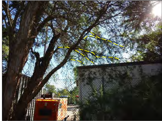
Photograph 5: Tree 4 Callistemon slaignus (Weeping Bottlebrush) to be selectively pruned to clear site sheds.
