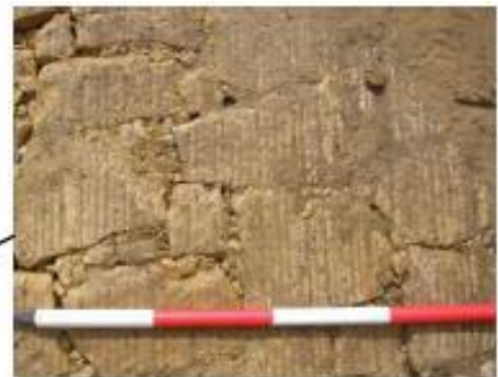
Figure 2: Close up detail of the sandstone surface showing material type, formation and construction detail. This is essential for establishing date of the feature.
